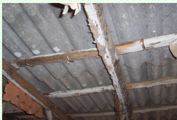
Rotting rafters to be replaced by Hope Abides. These support a roof over a dormitory for small children.
